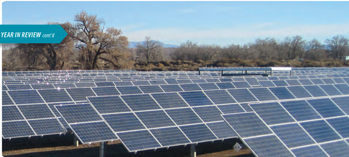
NAIOP, in giving the Water Authority its 2015 Vision Award, cited such environmental efforts as the solar array (above) at the utility's Southside Water Reclamation Plant.
