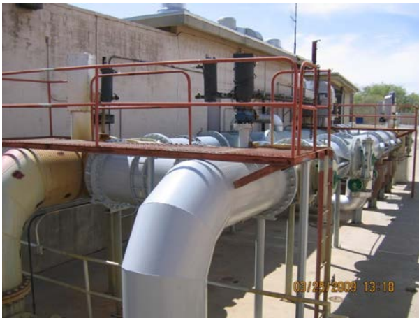
Lift Station #20 Force Main Header
