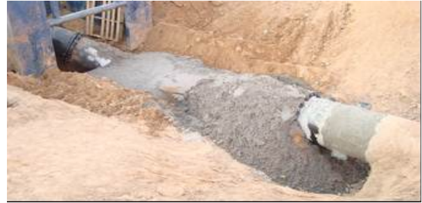
24" Concrete Cylinder Water Line
