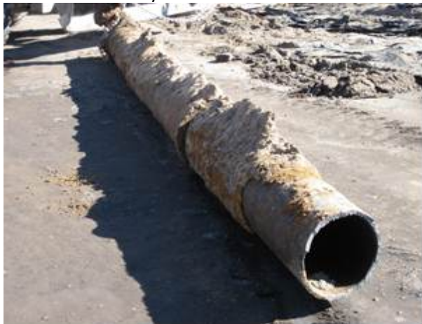
Corroded Steel Pipe
