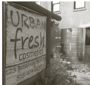
The 1,000-gallon rainwater collection system at Albuquerque's Urban Fresh Cosmetics.
