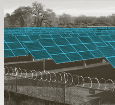
The solar array at the Southside Water Reclamation Plant is one of several environmental initiatives that have garnered attention for the Water Authority.
