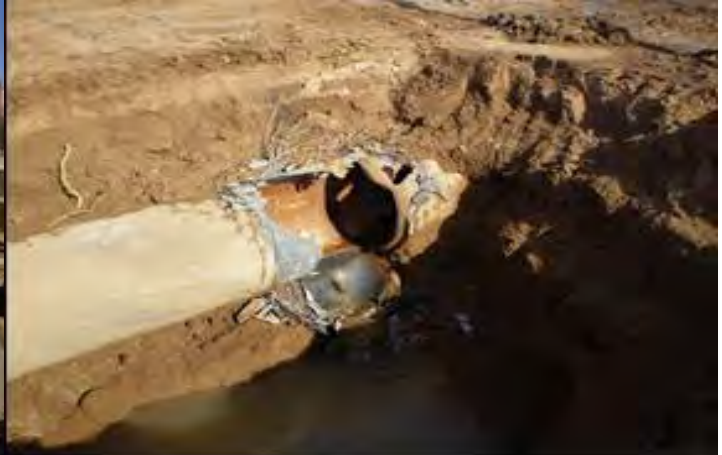
Valve to be replaced
