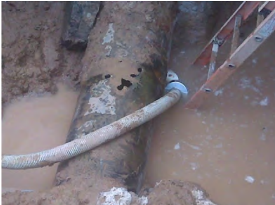
Hole in 20" Diameter Steel Water Line
