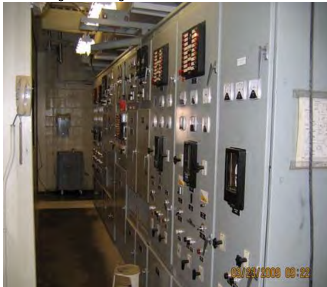
South Cogen Switchgear
