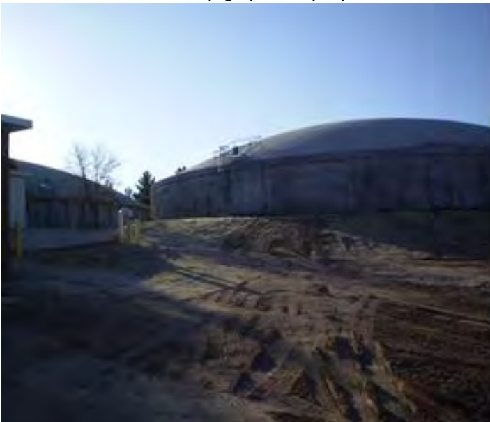
Lomas Reservoir Nos. 1 (right) and 2 (left).
