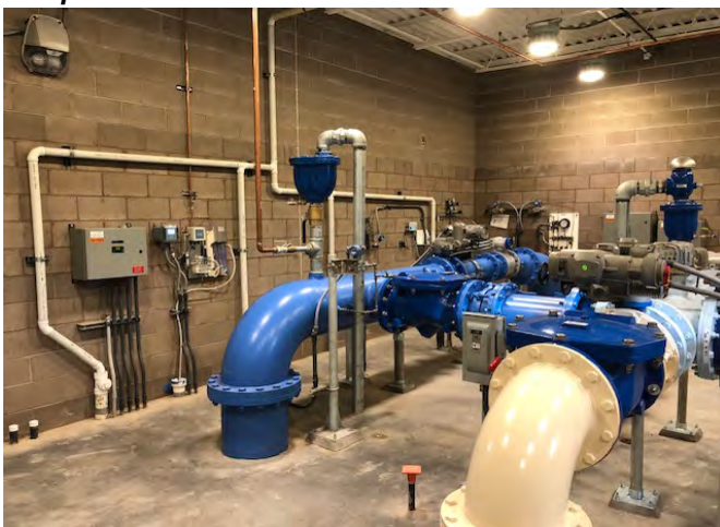
Deep ASR Well at SJCWTP
