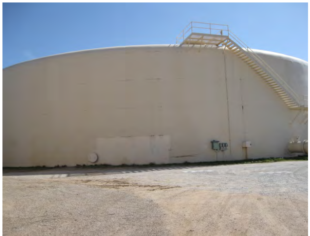
Coronado Reservoir - Steel Tank
