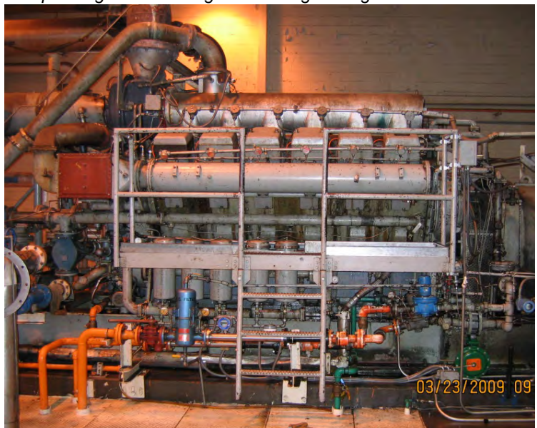
Cooper Cogeneration Engine at S.Cogen Bldg
