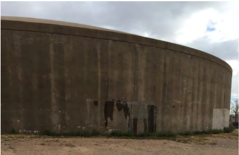
Duranes Reservoir with leaks
