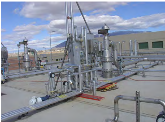
Ozone Monitoring Station Over Ozone Contactor Basins
