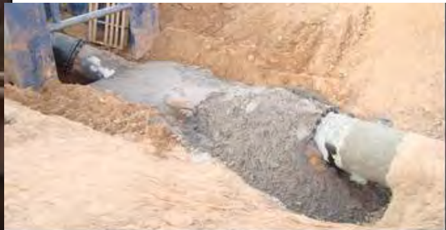
24" Concrete Cylinder Water Line Lowering and Relocation for a City Storm Drain Project in San Mateo NE
