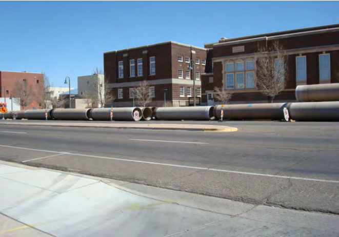
New 48” Sewer Line to be Slip-lined into an existing 54” Concrete Pipe in Broadway NE
