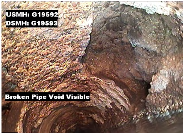
Sewer pipe with roof partially missing
