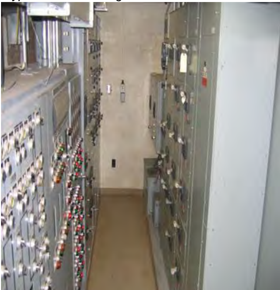
Typical MCC Switchgear
