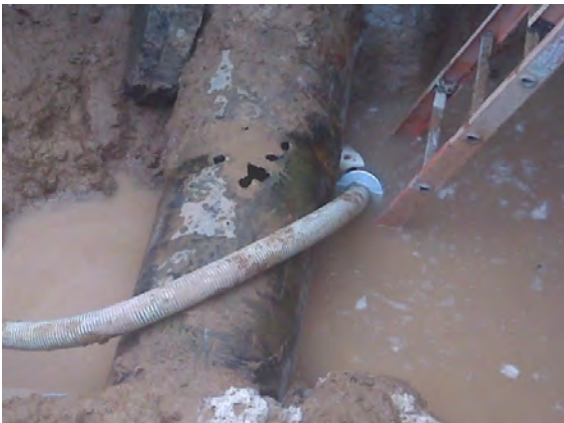
Hole in 20" Diameter Steel Water Line
