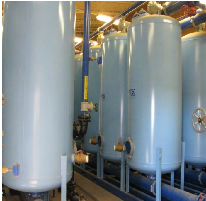
Corrales Well 3 - Arsenic Treatment System
