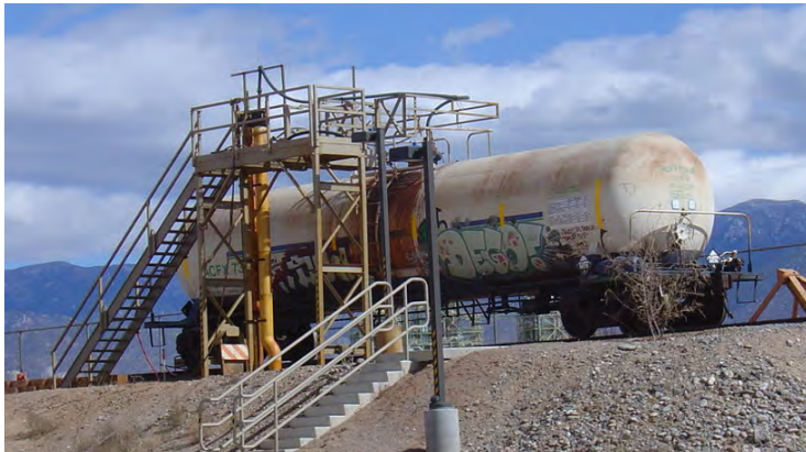
Ferric Chloride Railcar Unloading Station
