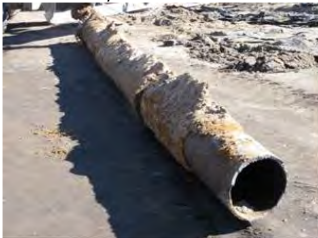
Corroded Steel Pipe
