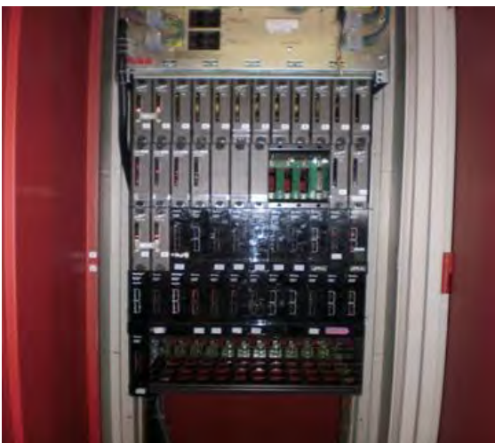
ABB Process Control Unit
