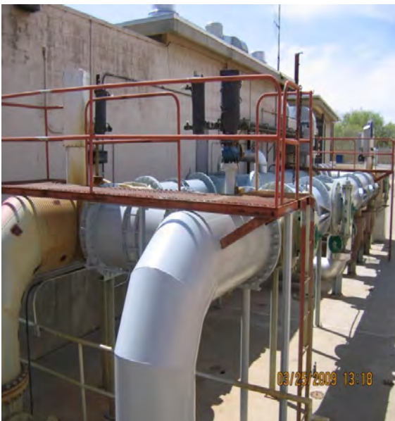
Lift Station #20 Force Main Header
