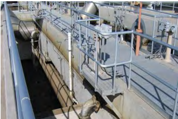
Aeration Tank Air Control Valve
