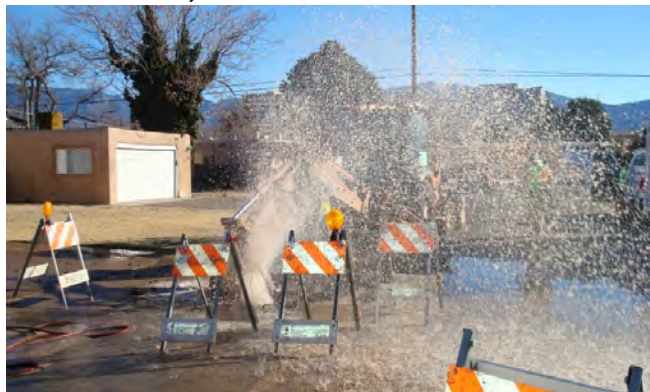
Steel line break, Hannett NE west of San Pedro
