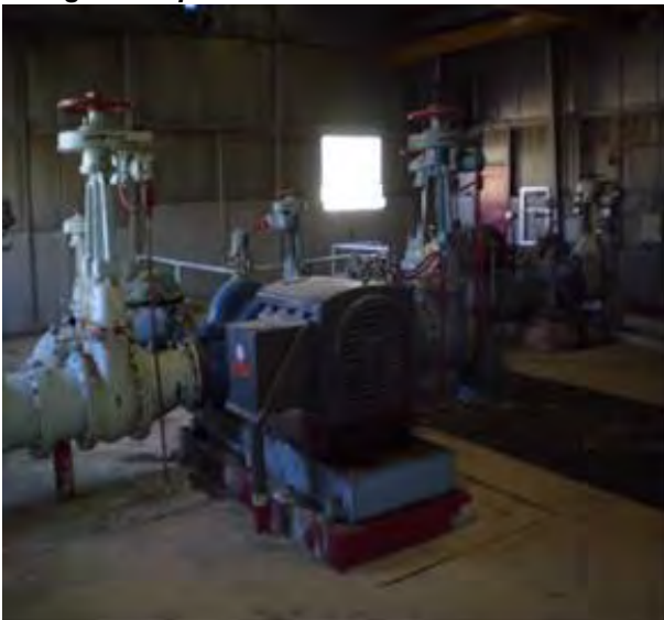
Griegos Pump Station - Interior
