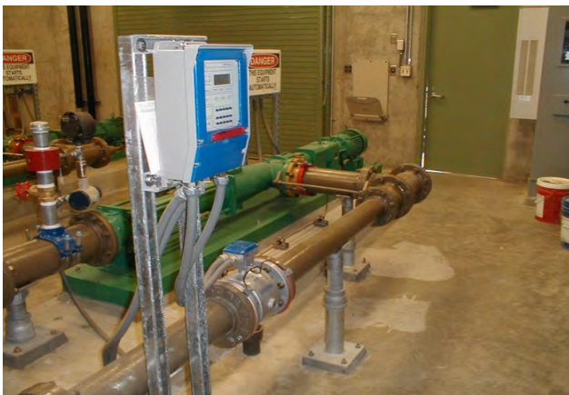
Progressive Cavity Sludge Pump at the WTP
