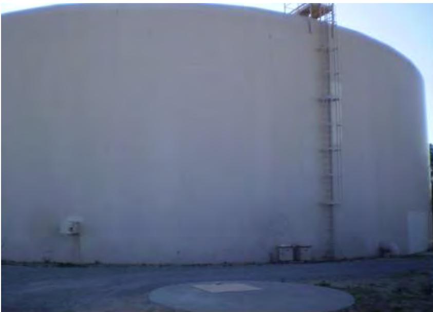
Santa Barbara Reservoir No. 1
