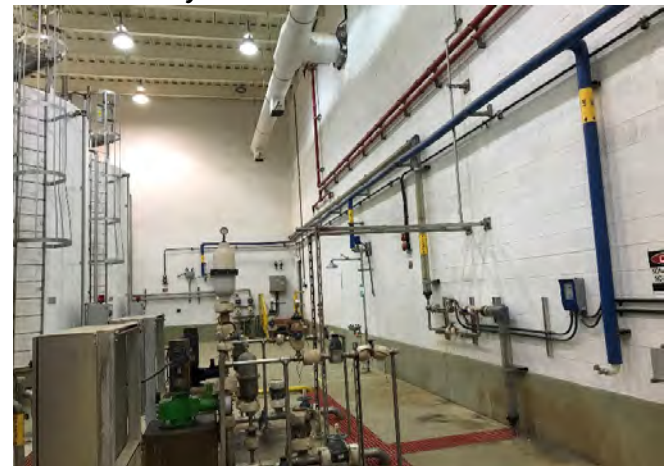
Sulfuric Acid System
