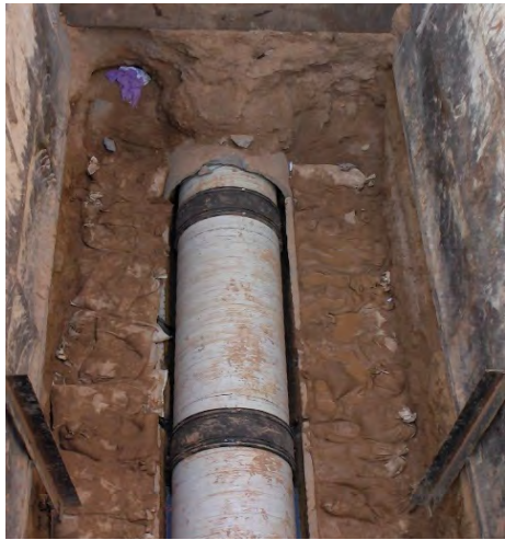
New 27-inch Sewer Line Sliplined in the old 30” Concrete Pipe in Prospect NE west of Carlisle
