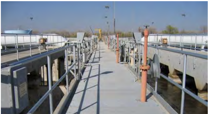
Aeration Tanks catwalk
