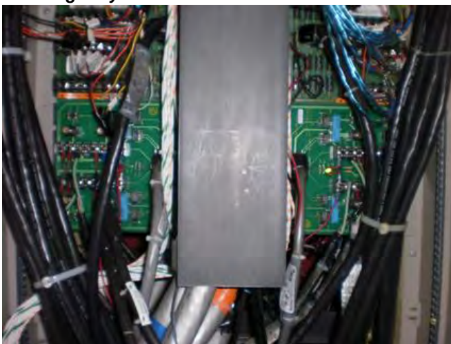
Data Highway Coaxial Cable Terminations
