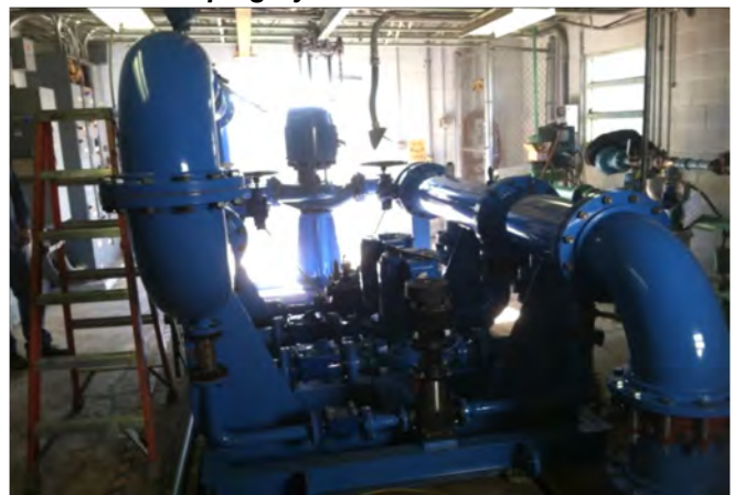
SAF Water Pumping System
