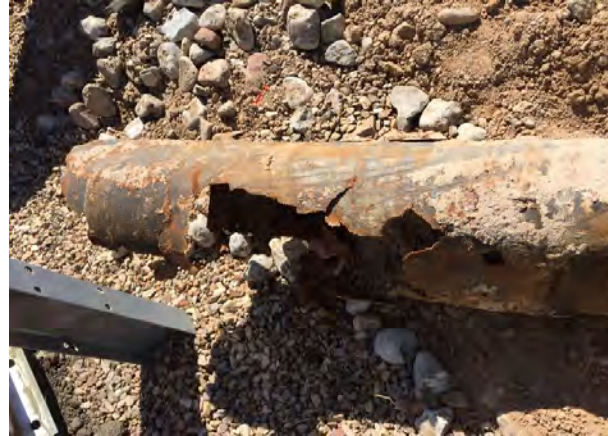
Severly corroded ductile iron sewer pipe
