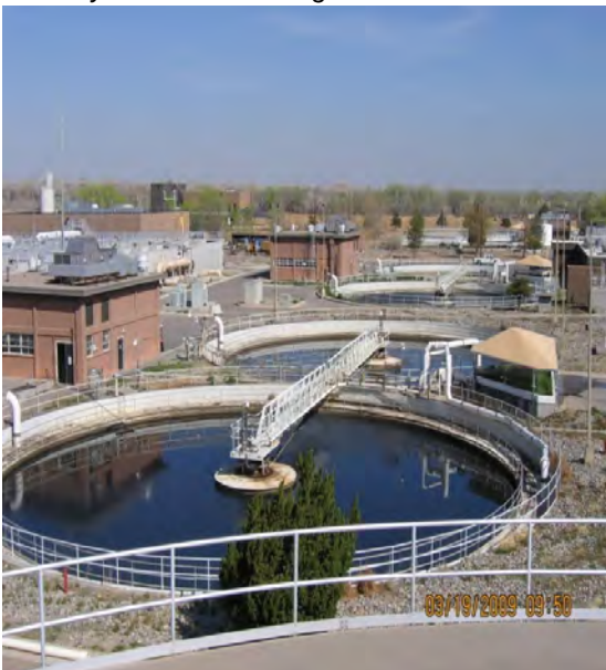
Primary Clarifiers 1 through 4
