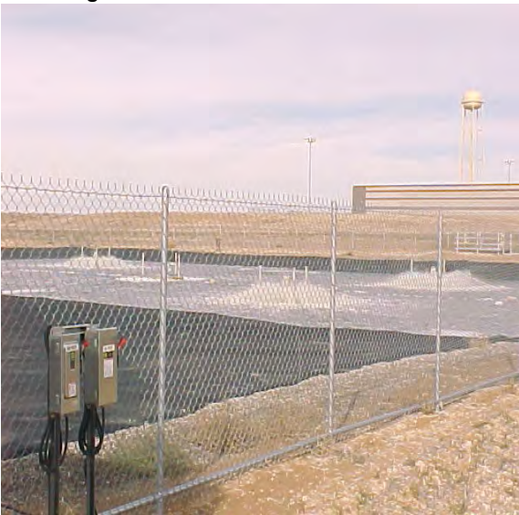
MDC Lagoon with Mixers and Aerators
