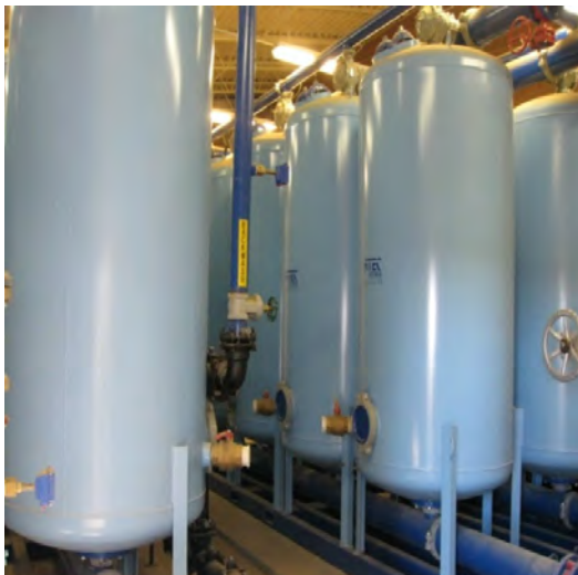
Corrales Well 3 - Arsenic Treatment System
