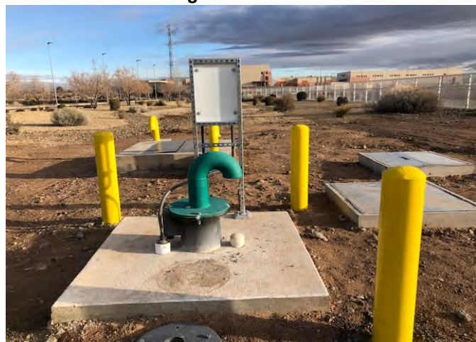
Vadose Zone Recharge Well at SJCWTP
