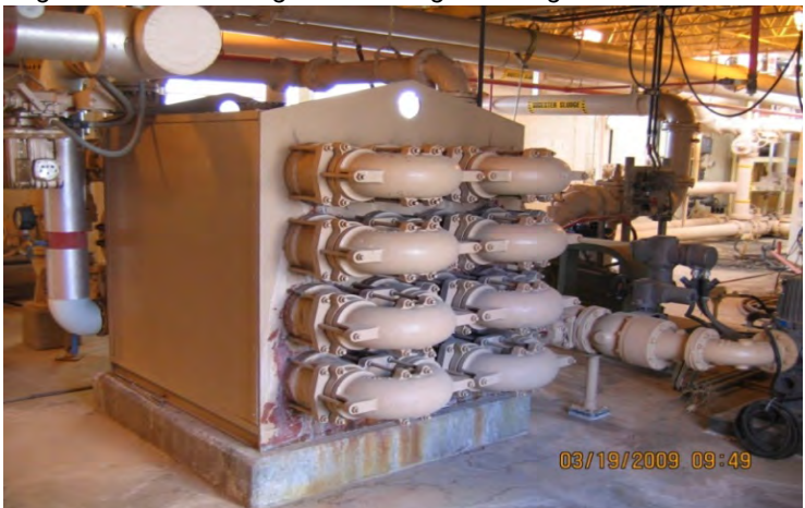
Digester Heat Exchanger for heating the sludge
